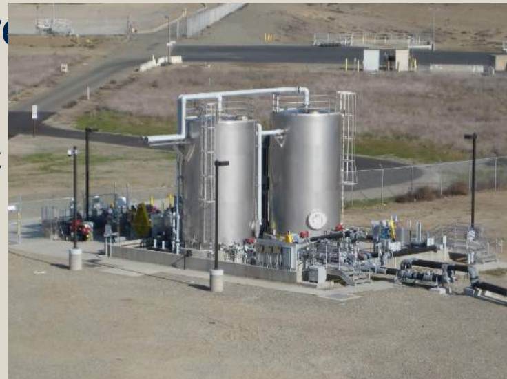
Biogas Enhancement Facility at Regional San's treatment plant
